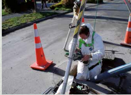
One of our technicians putting on their full face mask prior to repairing a leak in a manhole.
