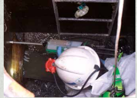
Technician fixing a leak by injecting through a manhole wall using a 'Quick Mix' cartridge system.
