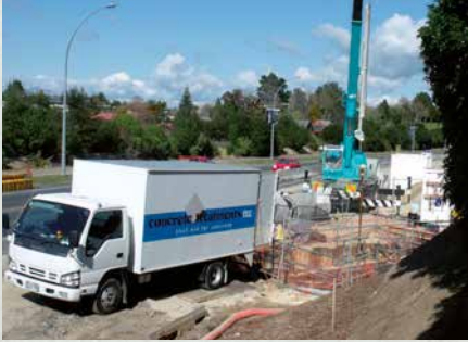
On site providing soil stabilisation inside a tunnel in Hamilton's running sands.
